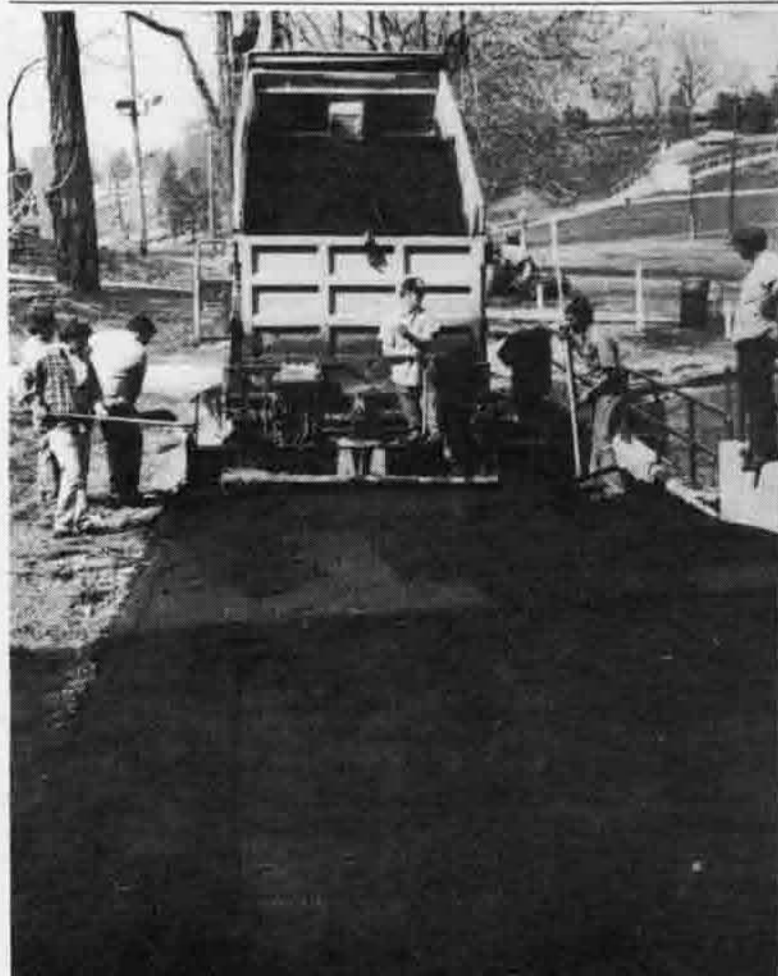
TARRED: Workers above tar a new path for UMSL students on the north side of the University Center [photo by Chuck Higdon].
